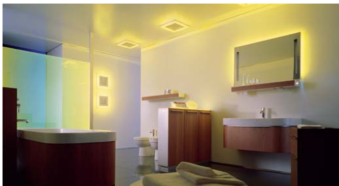
e stands for emotion: with different programmable lighting, the e-mood lighting system can be used to create different coloured-light moods.
